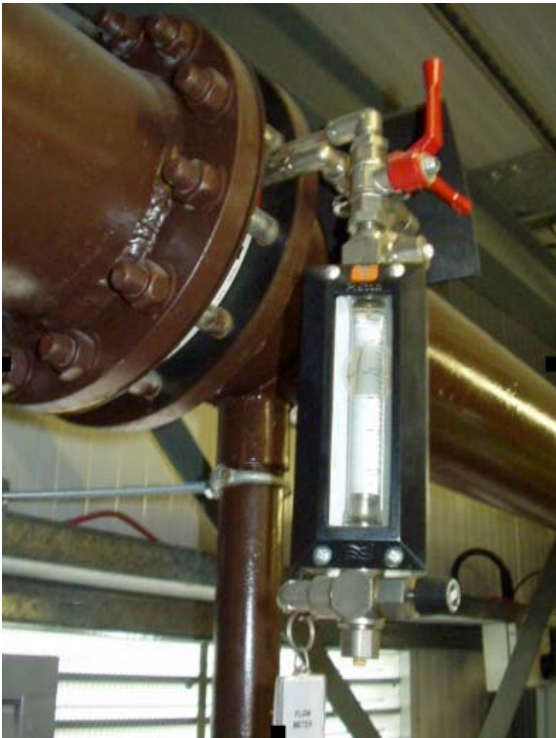
Flow test meter
