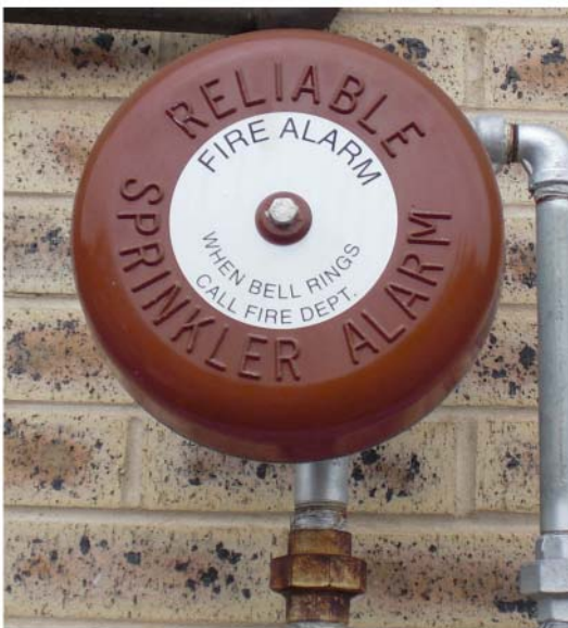
Hydraulic Alarm Gong
