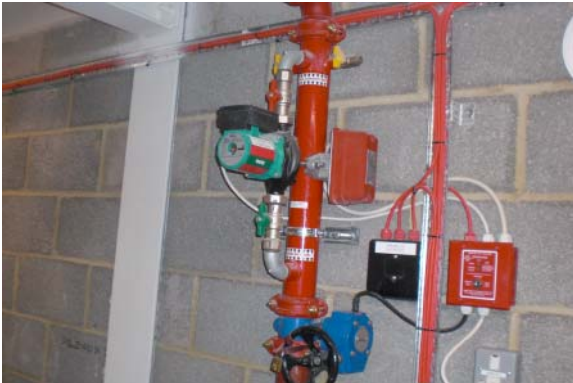
Tenants zone isolating valve with “zonecheck” flow switch test device.
