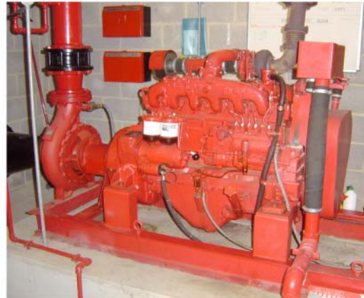
Diesel engine driven fire pump
