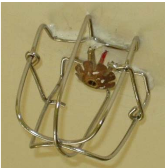
Sprinkler head fouled by plaster
